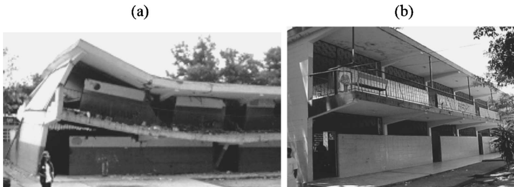
Figure 9. Old-type school buildings: (a) VV school that collapsed in Cariaco; (b) identical buildings can be found in several locations in the country.
